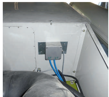
Differential pressure sensor records measured values, and relays them to the measurement box.
