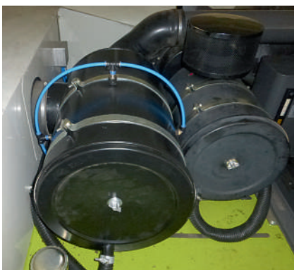
Piezometer ring on the air filter housing measures the differential pressure before the filter.
