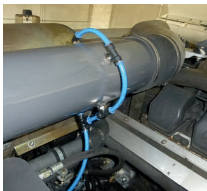
Piezometer ring on the air baffle measures the differential pressure after the filter.
